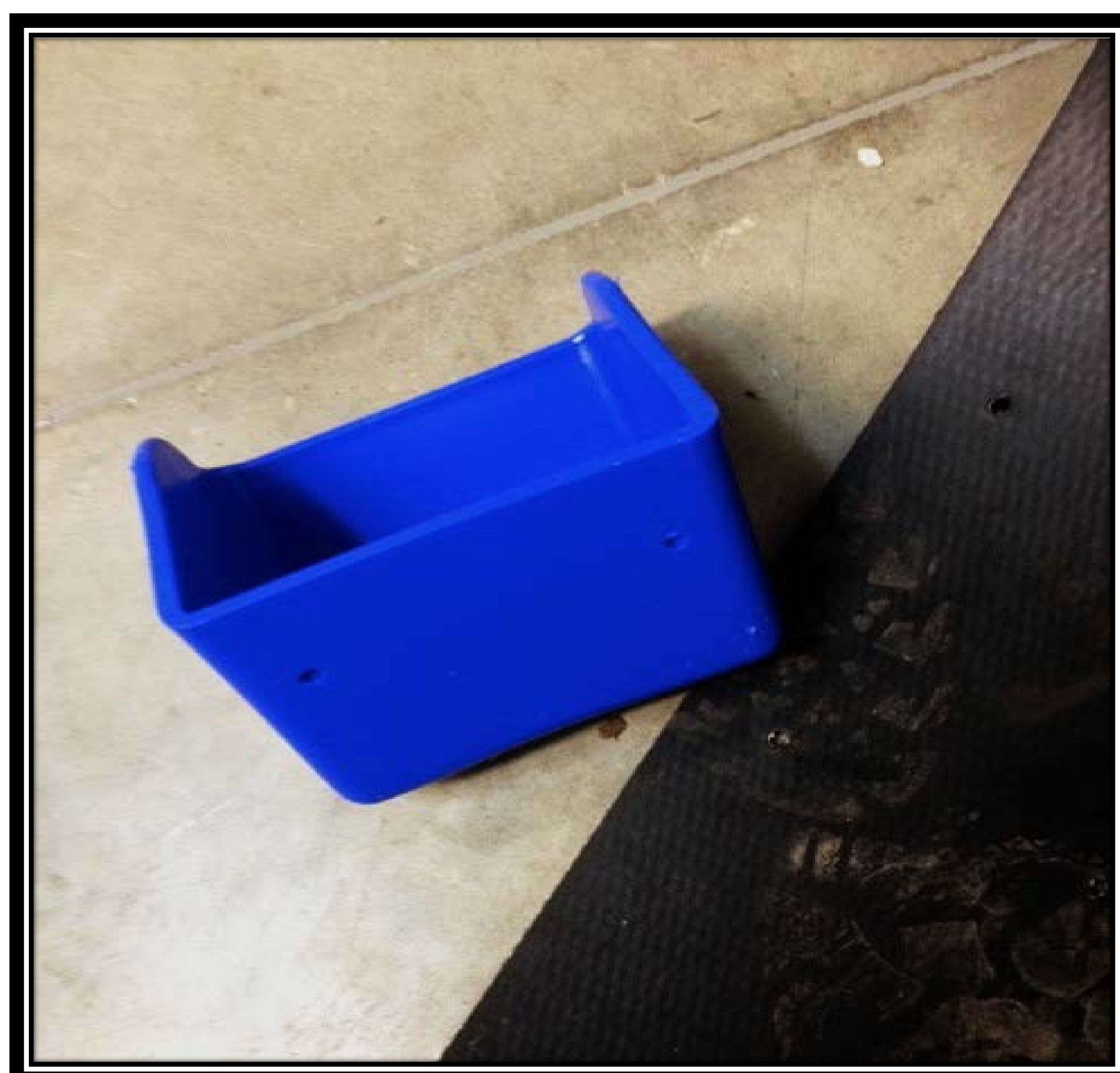
Pictured here are a bucket and a piece of the belt. There are 110 buckets inside the leg attached to 28' of belt.
